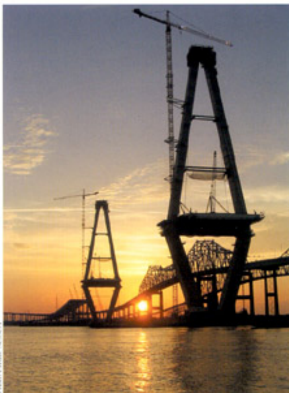
The true form of the diamond towers emerges from the construction process.
