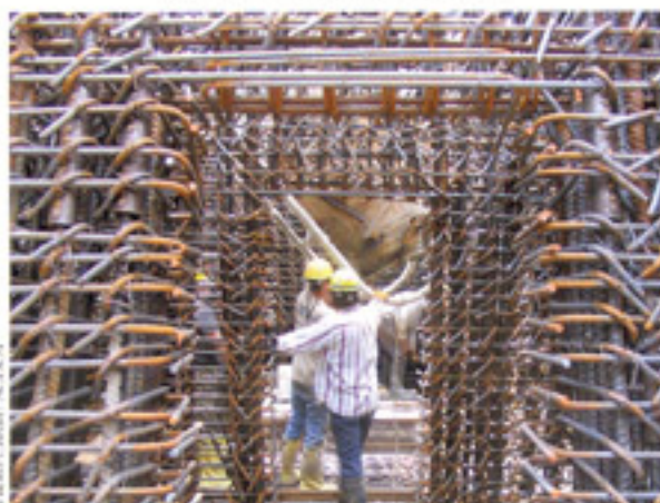
Massive amounts of re-bar designed by the structural engineer will be concealed by the form of the concrete envisioned by the architect.
